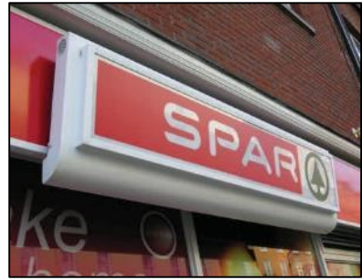
Figure 152 - NO - New, internally-lit, plastic signs are not appropriate on historic buildings.
